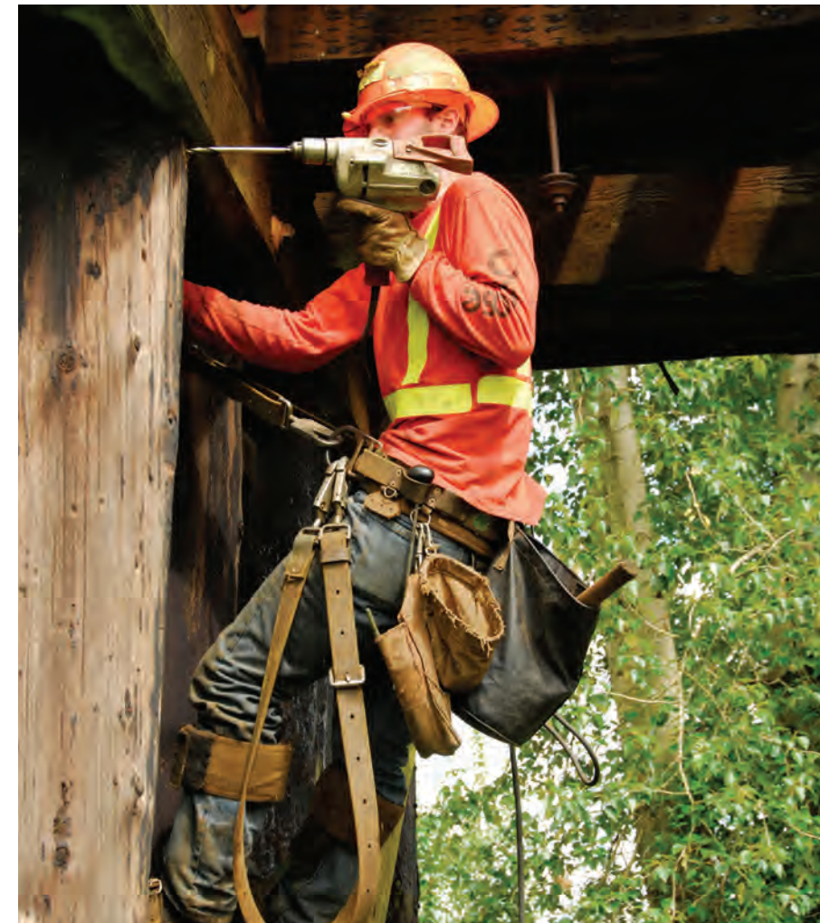
Osmose obtained detailed information on the piling, caps and stringers using the company’s proven methods of hammer sounding, boring and quantifying the results by measuring shell and void in the timber members.
