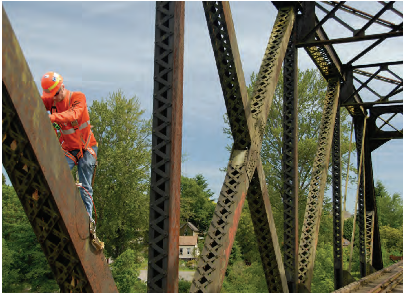
Osmose points out that the inspection of a steel thru truss is not accurate unless you actually physically climb over the upper chords and underneath the bottom chords. Corrosion, missing rivets and crack identification are key priorities during the steel inspection.
