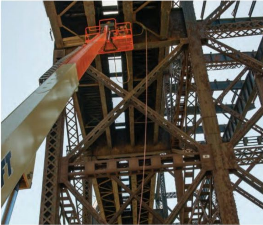
THIS PAGE: An inspector looks at the underside of one of the TRRA's bridges.
